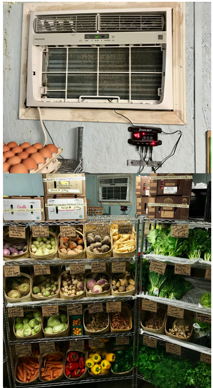
Photo 3.3. Swamp Rabbit Cafe and Grocery's Produce Room with an A/C unit and CoolBot® controller.
