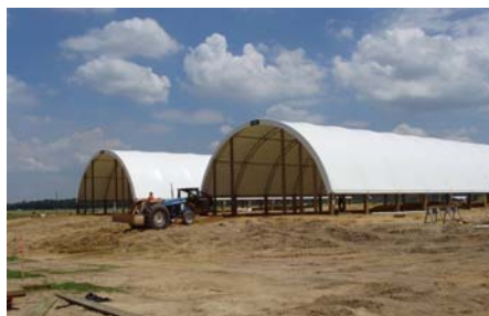
Above: Construction of hoop house frames; below: hoop houses after addition of the roof cover.
